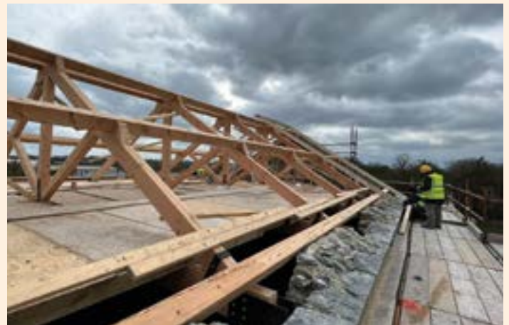
Construction taking place on the roof of the events and hospitality building
