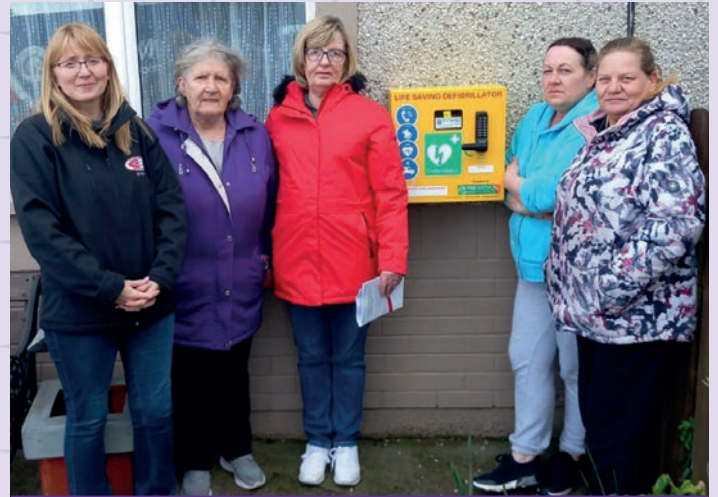
St Theresa's, St Anns, St Grellans Residents thanked all those who took part in our fundraising drive to buy and install their own Defibrillator at 18 St Grellans Tce. It was installed by Oliver Mullen Electrical contractor.
